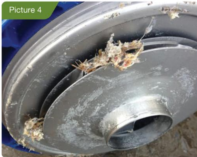
Pump Impeller blocked by debris.
