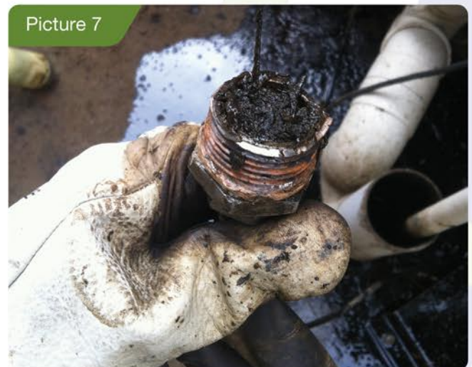
Equipment blockages due to rubbish.
