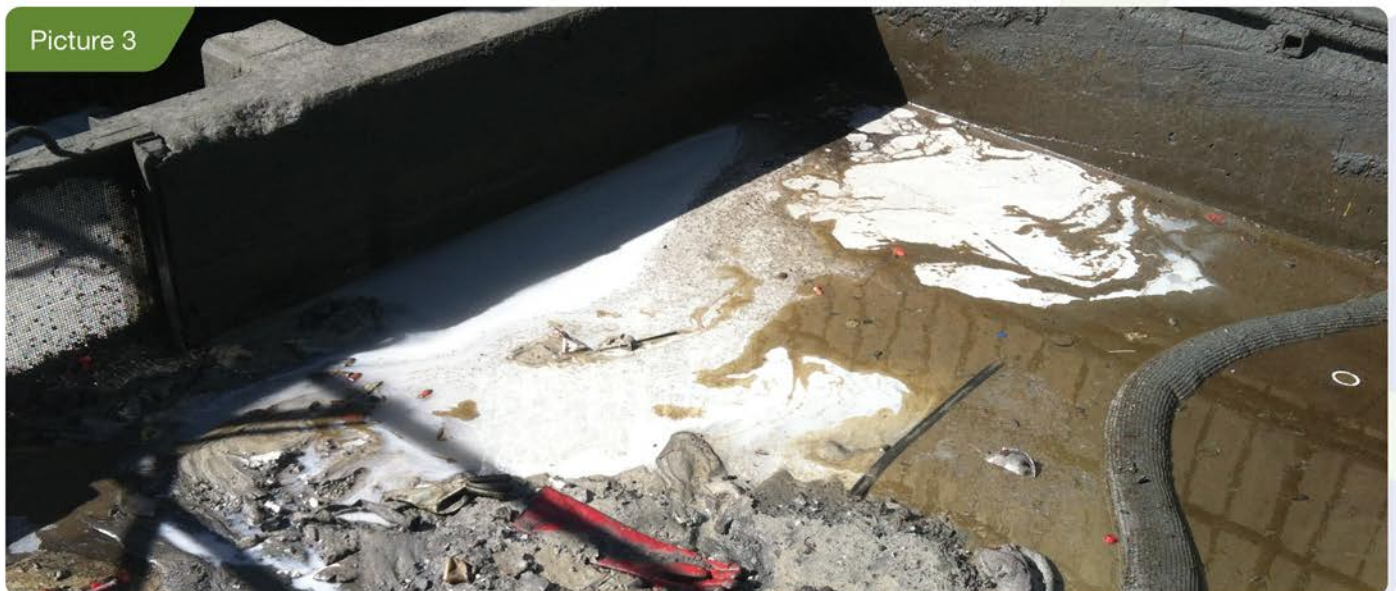
Trash & debris in oily water collection pit.
