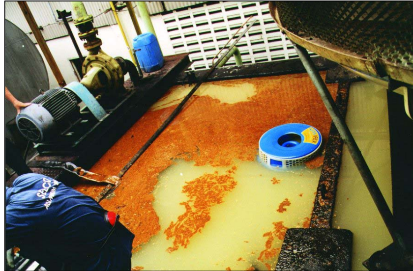
Pictures of water sample and hot & cold wells before installation of Ultraspin system.
